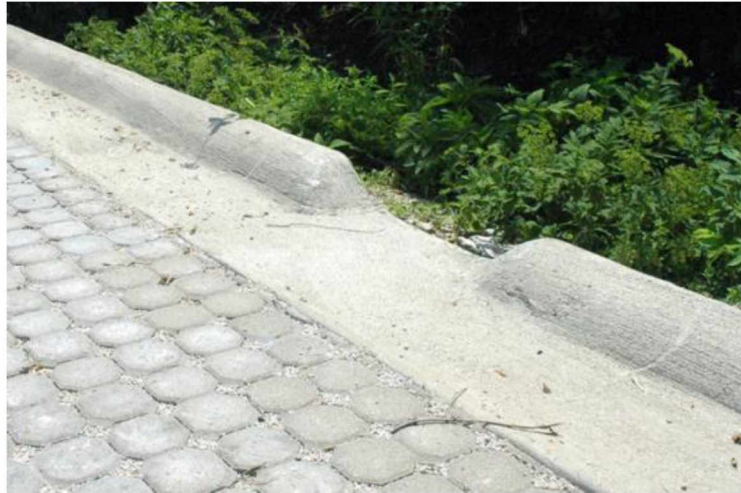
Figure 3: Cuts in the continuous curb allow for stormwater to be directed into landscaped areas
